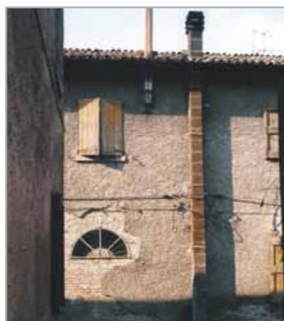
Fig. 5.3 - Wall with rising damp
