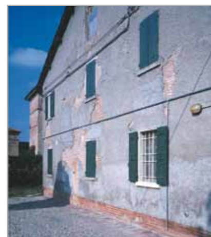
Fig. 5.4 - The areas of loose render must be removed before bonding the insulating panel
