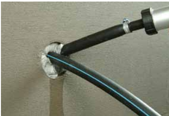
Then KÖSTER KB-Flex 200 is filled into the void using the KÖSTER Special Caulking Gun.
