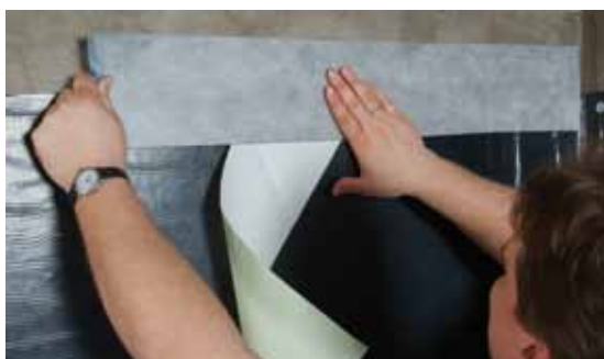
If no separate base waterproofing is installed, the upper edge of the waterproofing layer has to end approx. 30 cm above grade. In order to achieve an attractive visual appearance, the upper edge of the membrane can be covered with the cold self-adhesive KÖSTER Butyl Fix-Tape Fleece. This tape can be plastered over.
