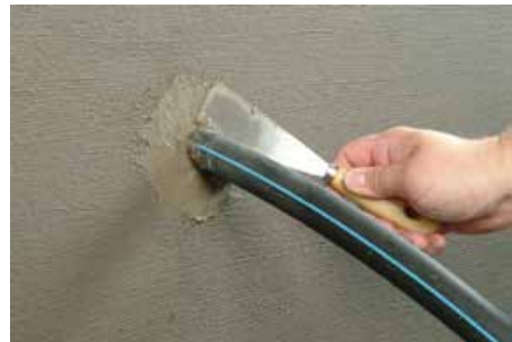
The pipe penetration is now waterproof. In order to protect the waterproofing the area around the pipe or cable is plugged with KÖSTER KB-Fix 5.
