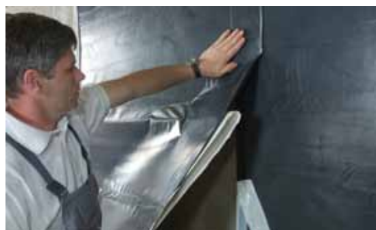
The area is waterproofed with the membrane. Membranes must overlap by approx. 10 cm.
