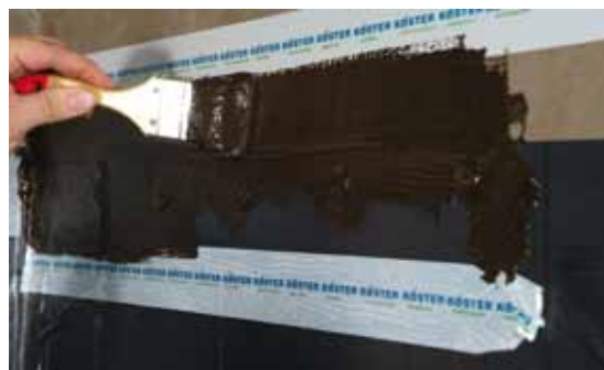
The edges of the membrane are sealed with KÖSTER KBE Liquid Film.
