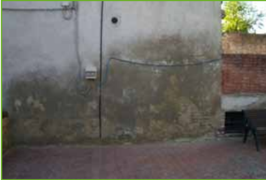
Change of colour, reduction of the thermal insulation.
