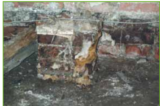
Development of mould and damage to the fabric of the structure
