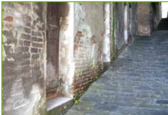
Destruction of render and mortar joints
