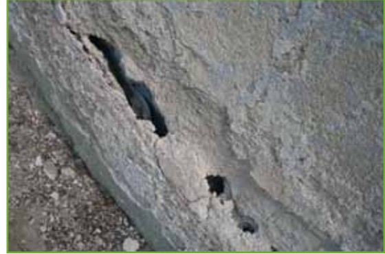
Damaged plaster / render
