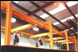
OVER HEAD CRANES
