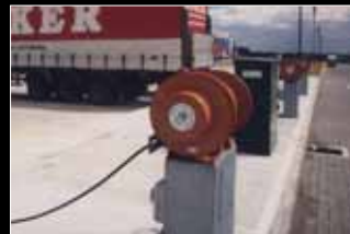
CABLE/HOSE REELING DRUMS
