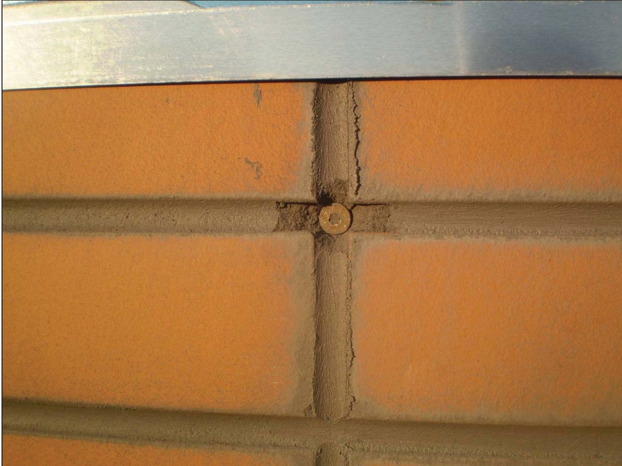
GEBRIK FIXING SCREW REVEALED AFTER 500 NM IMPACT
