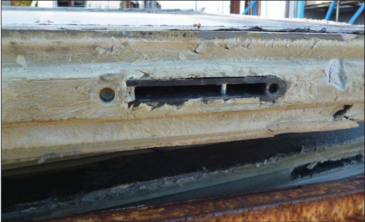
SIDE OF UPPER COMPOSITE PANEL REMOVED FROM TEST RIG
