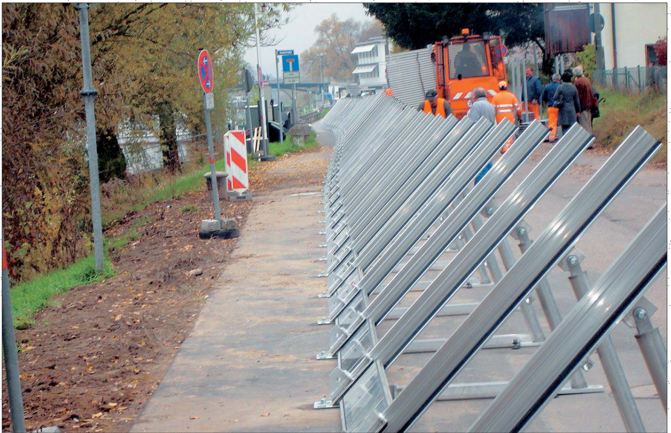
Fastening possibility: K-trestle bolted with water-sided peg fixed into the street ground surface
