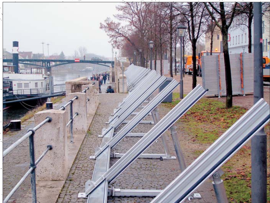
IBS system in the construction stage of K-trestles and the first dam beam with ground seal
