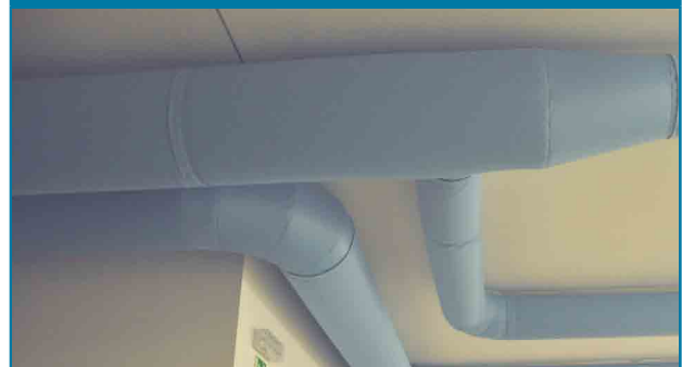
Air transfer ducting
