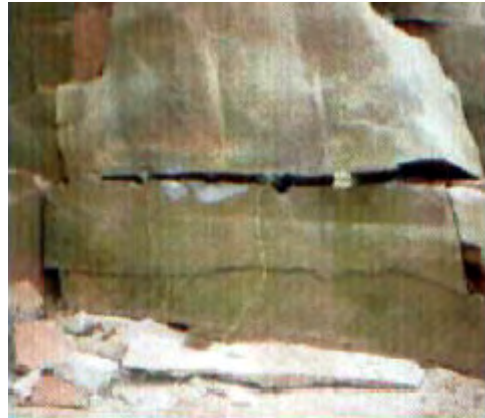
CARDOX Tubes applied horizontally to lift a block along its natural bed plane.
