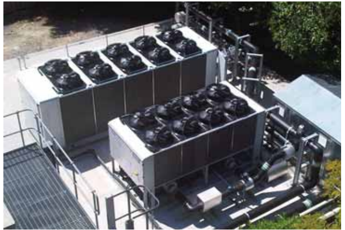
IBM data centre
