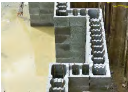
STEPOC in a basement level application
