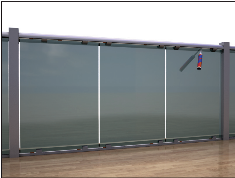
47 Apply a thick bead of high quality silicone sealant to continuously fill the gap between top of glass and handrail
