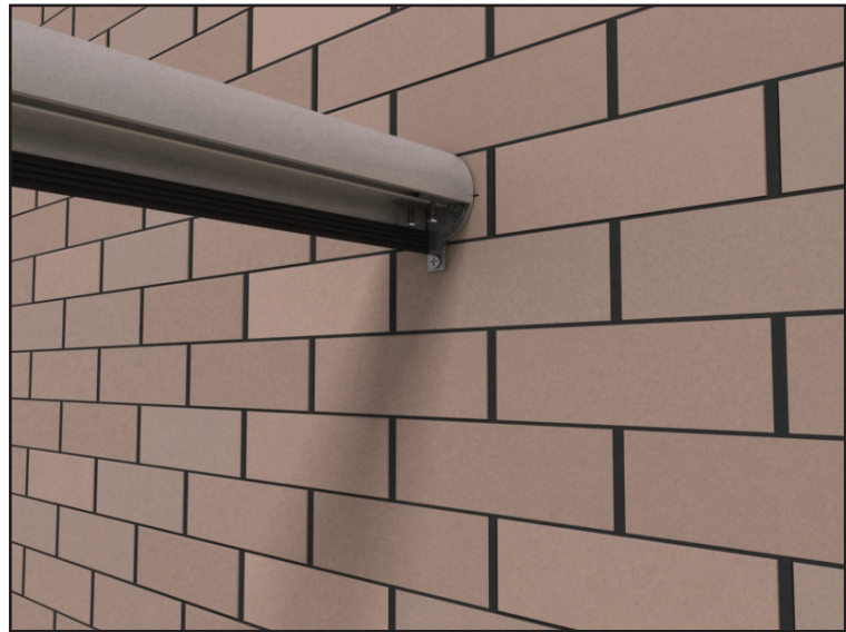
27 Drill 4mm holes through brackets in the handrail. Fix the handrail to the wall bracket using the No. 10 x 3/4" S/tapping screws
