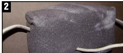
2 Insert cables through the cover. Hold onto the string to prevent the cover from falling into the cavity. Picture shows view from inside the cavity, where several cables have been inserted into the cover.
