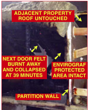
AFTER THE FIRE TEST
