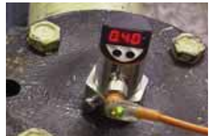
Local display: the clearly readable LED display shows the current system pressure.
