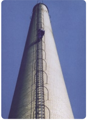
Chimney with retrofitted guide rail
