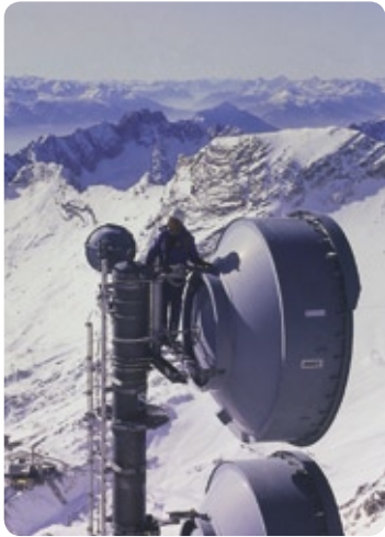
Telecom-station with aluminium ladder on the Zugspitze
