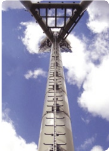
Floodlight mast for stadium lighting with galvanized steel ladder
