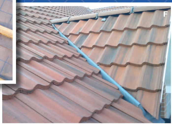
F. The completed installation: neat, tidy and effective – with minimal on-site time.
