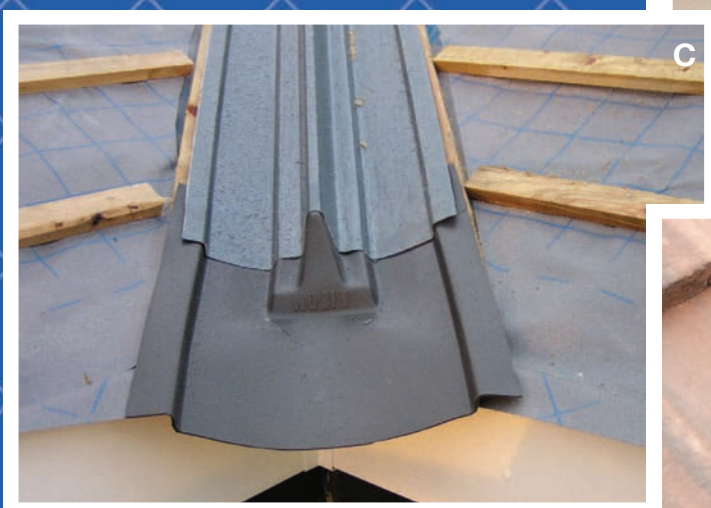
C. The V-Flow DF valley trough is fixed in position over the eaves closure piece at 50 mm centres, with large headed galvanised or aluminium nails.
