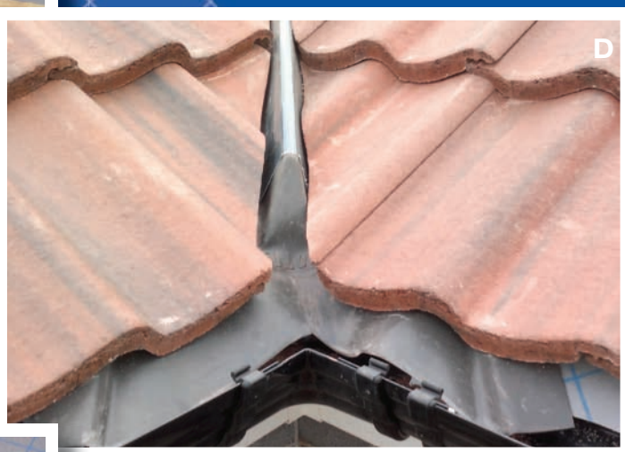
D. The eaves closure piece is cut to allow water discharge into the gutter.
