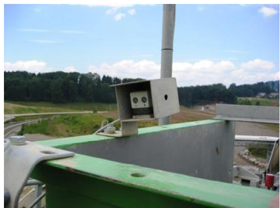
Ultrasonic sensor in the transfer hopper
