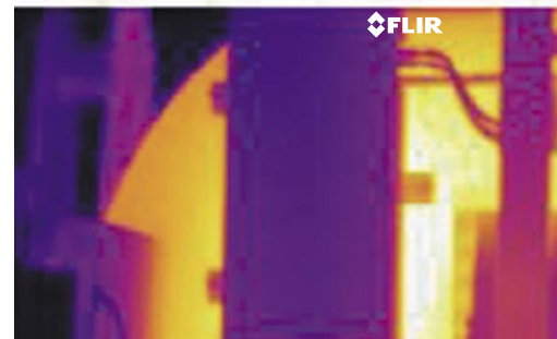
Infrared picture of a ladle slide gate in the ladle make up area. The infrared picture shows the hot ladle bottom under the slide gate.
