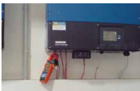
These inverters convert the direct current from the solar panels to alternating current.
