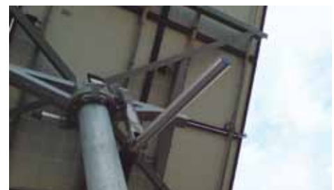
Inspection from the back shows no hot spots, the hot spots in the previous thermal image taken from the front were caused by reflection.
