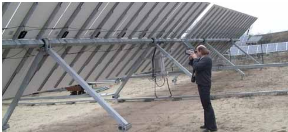
Volker Denzler, thermography expert at SOLON's after sales services department, takes thermal images from the back of a module to avoid reflections.
