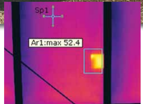
This thermal image shows a hot spot due to cell breakage in a standard 60 cell module.
