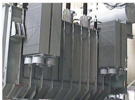
▼ A 225 MVA transformer
