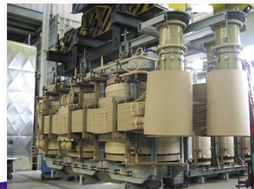
▼ The interior of a 225 MVA transformer: reels and cables are covered with cardboard
