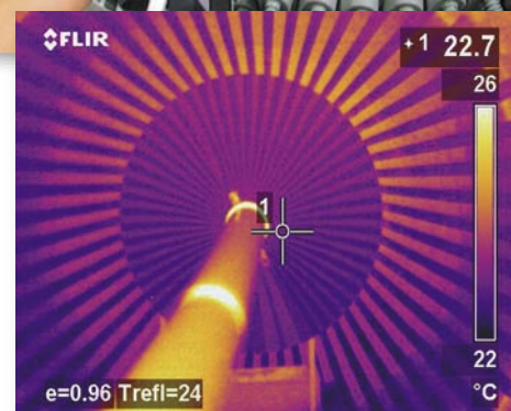
Generator stator core flux test; ThermaCAM™ S60 proves integrity of stator core plates
