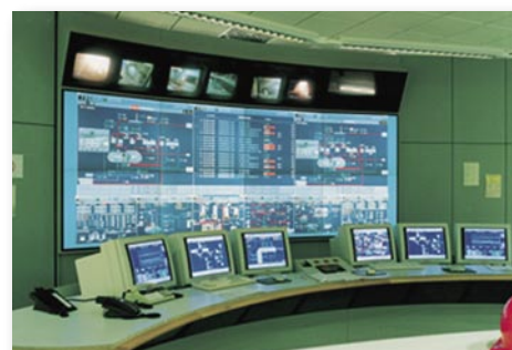
The control room of a waste bunker. If the ThermoVision™ A40 detects a hot spot an alarm will go off.
