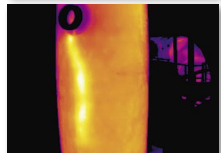
Failure in internal refractory lining
