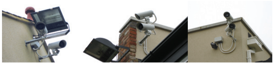
These six FLIR SR-313 thermal imaging cameras cover the back of the estate
