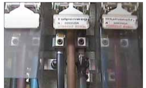
This connector has become resistive due to loosening and corrosion. This can be easily remedied by opening, cleaning and reassembling the connector.
