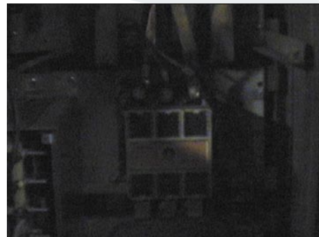
Checking the main switch inside an electrical panel
