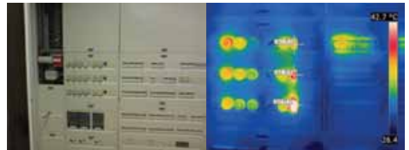
This thermal image shows that the work load during operation is not distributed evenly among the fuse boxes.
