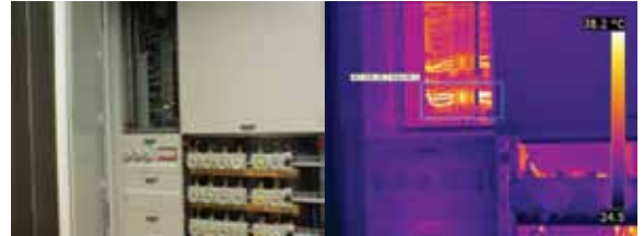
Although these output terminals are definitely hot, the measured temperatures are normal for this kind of load.
