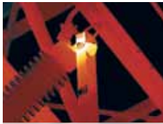
Incorrectly secured connection
