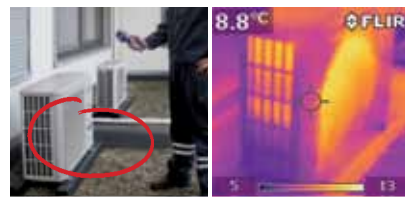
Check-up of an air conditioning installation quick and easy.
