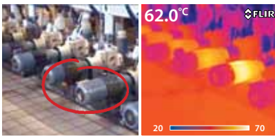
Mechanical check-up of an electrical motor using the FLIR E-Series.
