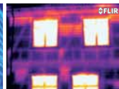
Framework construction. Many of the sections are missing insulation as indicated by the warmer colors.
