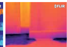
Moisture intrusion in floor, impossible to see with the human eye, but clearly visible in the thermal image.
