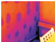
The thermal image shows mould on the interior wall due to water infiltration.
