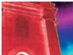
The thermal imaging reveals a hidden window construction invisible to the human eye.
