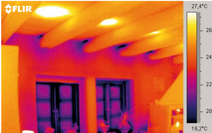
Here, the bridging is between the roof beams and the adjacent wall.
