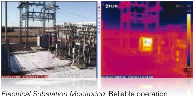
Figure 10. Visible light and IR images of a substation showing a transformer with excessive temperature.
