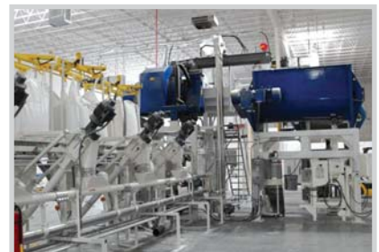
An AMC with multiple inlets delivering cement, sand, ash and recycled glass to a second unit that lifts them up into a mixer.
