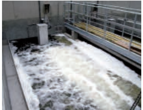
VRM® unit in operation
