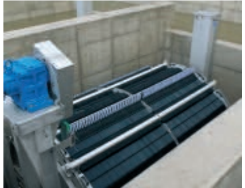
VRM® 30 filtration unit installed in the filtration chamber
