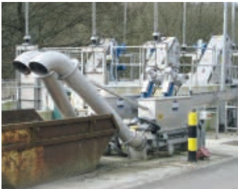
Redundant operation and optimal screenings dewatering with launder channel feeding system
