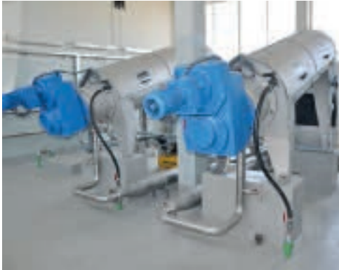
Two RoS 3Q Screw Press units installed in parallel
