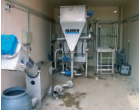
HUBER ROTAMAT® Micro Strainer with 1 mm bar spacing and HUBER Dissolved Air Flotation Plant HDF
