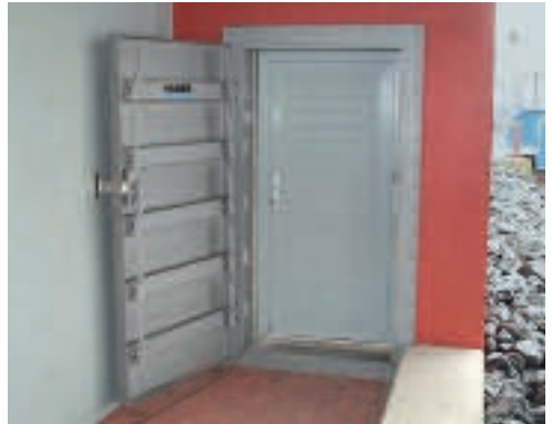
Pressure door installed for flood protection
