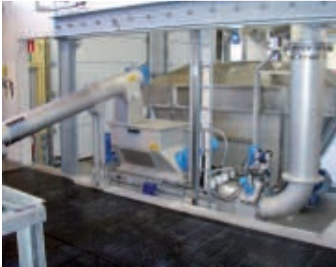
Best screenings washing and compression in a single unit
