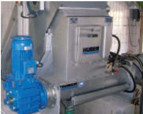
HUBER Screenings Wash Press WAP installed behind a STEP SCREEN®
