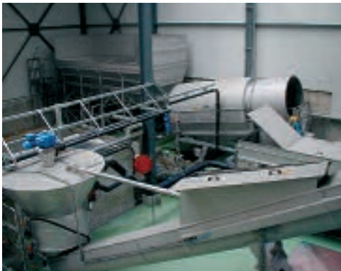
HUBER Grit Treatment System RoSF 5 in Cridec, Switzerland
