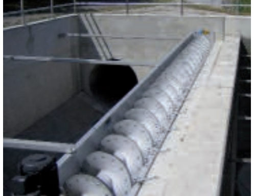
ROTAMAT® Storm Screen RoK 1 installed on dry side of overflow weir
